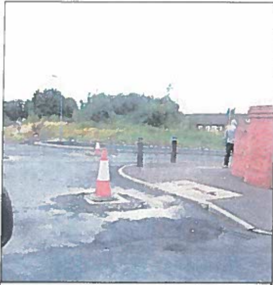
Taken During District Valuer's Inspection – Whilst very advanced some limited work remains to be completed
